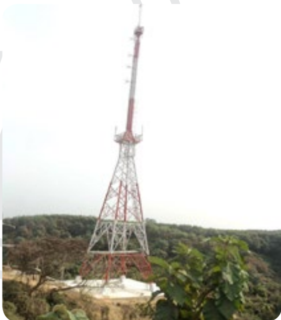
50 m tower installed at Udaipur site, distt. Agartala, Tripura state installed by TCIL in 2015
